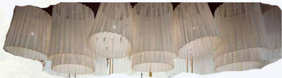
Ceiling hung fixture
