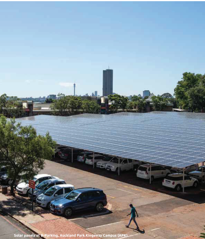
Solar panels at B-Parking, Auckland Park Kingsway Campus (APK)
